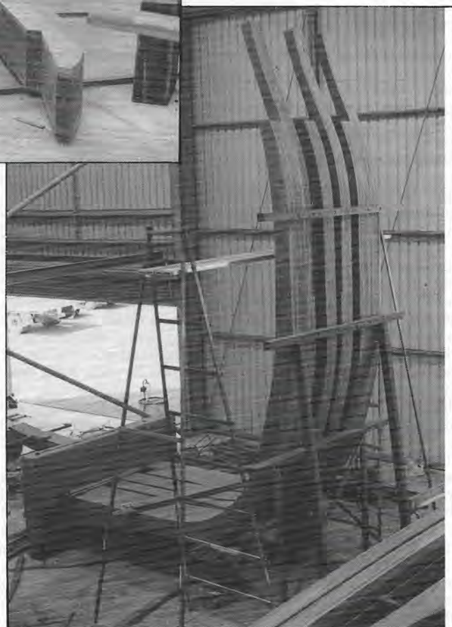
BUILDER Steve Ward is constructing the replica of ENDEAVOUR at an acceptable level of authenticity where possible, using traditional shipbuilding techniques but making use of modern machinery and fastenings to pre-fabricate floors and frames in his factory. Hull will be assembled on the Fremantle foreshore where public will be able to view this historic replica being built including mock-up to show frames of hull, pictured at left. (Peter Campbell pics).
