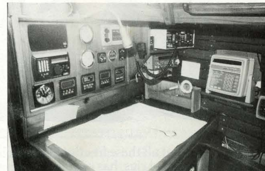
Navigation area with complete array of electronics, including Magnavox satnav, B&G Hercules instrumentation, B&G Homer RDF, two SSB radios.
